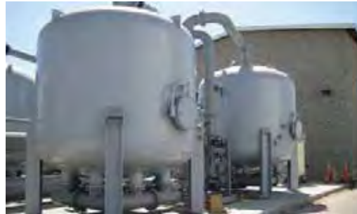
Figure 4-10: Vessels Utilized in the Perchlorate Ion Exchange Treatment Process
