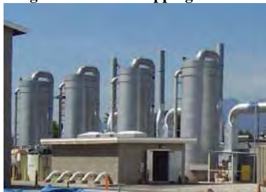
Figure 4-8: Air Stripping Towers
